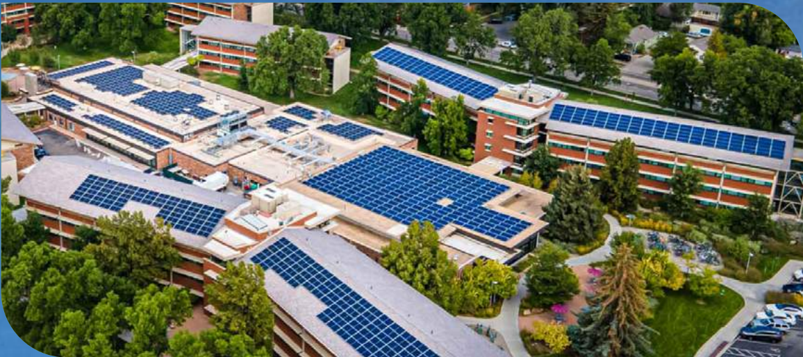
Installation at Parmalee and Corbett residential halls, and Laurel Village Complex at CSU
